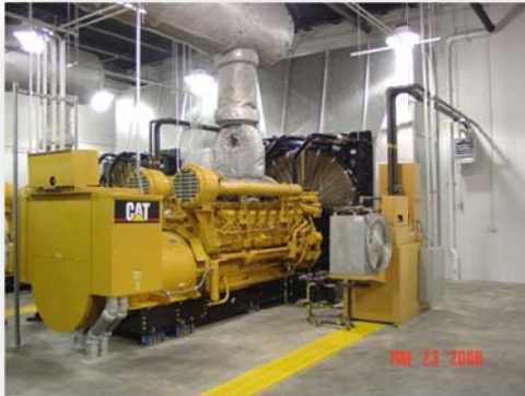
New electrical generator built in 2006
