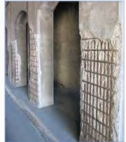
Many of the railroad overpasses downtown require attention.
